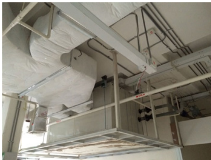
Air Handling Unit Copyright: www.123rf.com
